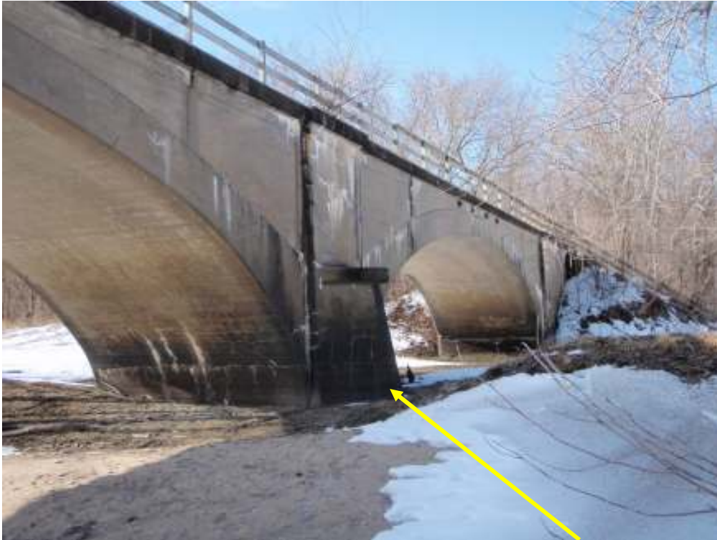
West end of McFarlane Bridge showing triangular pier abutment to protect bridge from ice and debris
