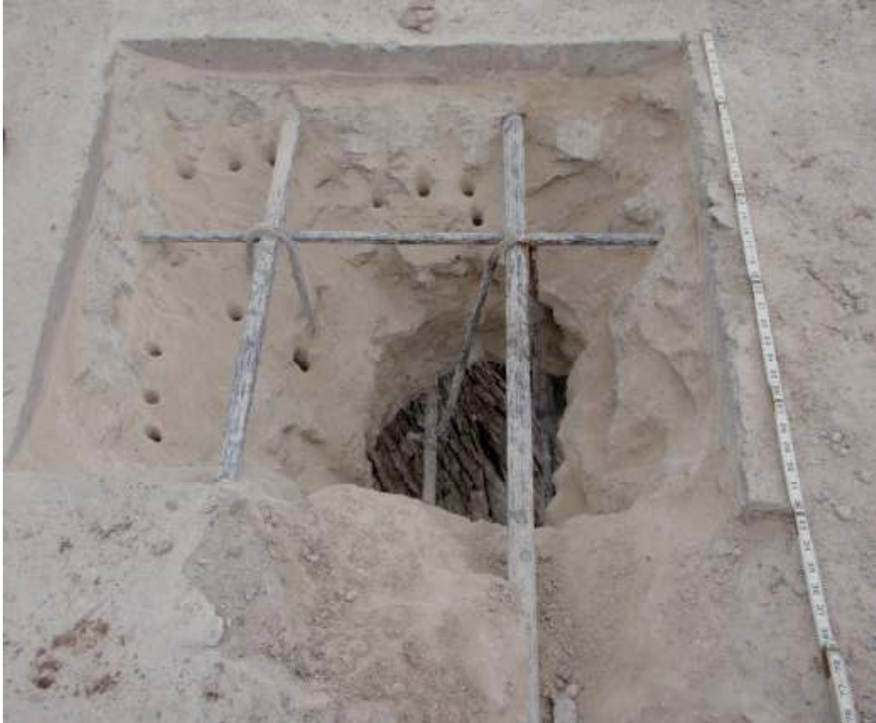
Looking down at the test pit excavation exposing reinforced bars on one of the arches on the McFarlane Bridge. Note the center hole punched down entirely through the arch, with tree debris in the river below visible through the hole.
