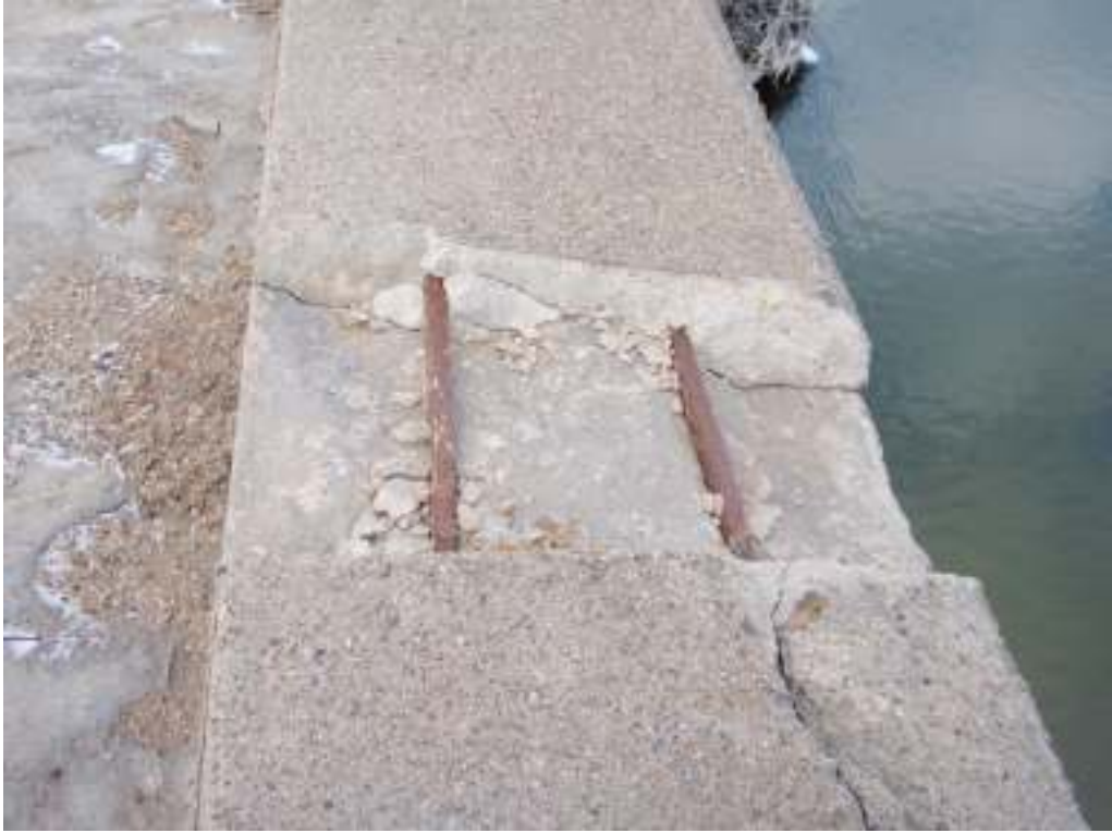
Detail of railing on McFarlane Bridge showing erosion exposure of reinforced bars
