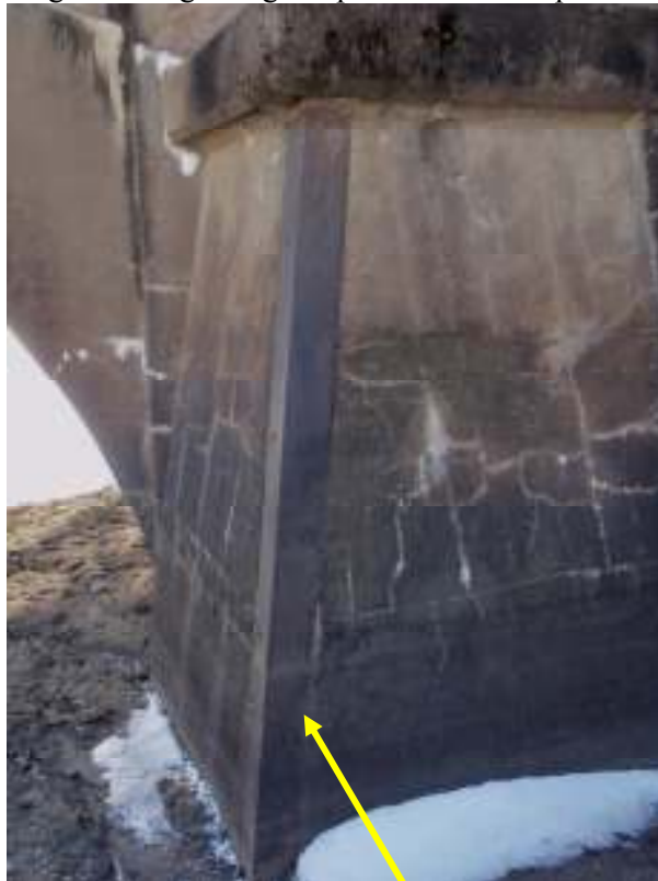
Detail of triangular abutment with cast iron plate to protect from ice and debris
