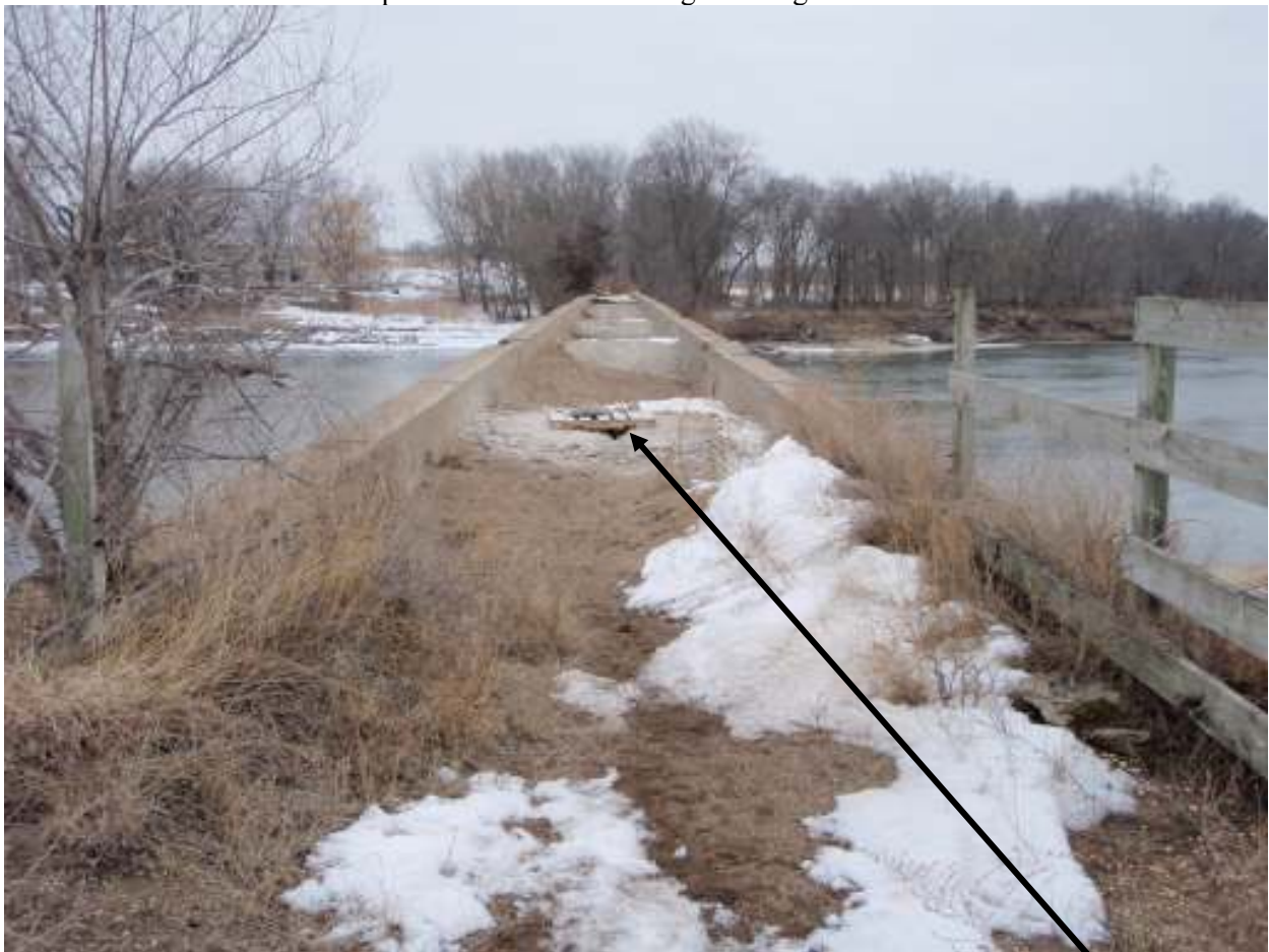
Top side of McFarlane Bridge looking to the ESE from near west end and showing test pit location
