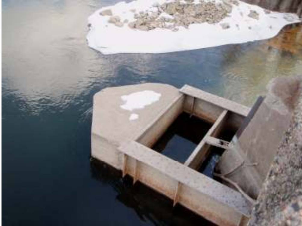
Caisson added to north side of east pier of McFarlane Bridge in the 1950s following subsidence
