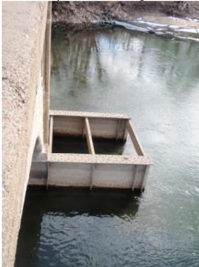
Caisson added to south side of east pier of McFarlane Bridge in the 1950s following subsidence
