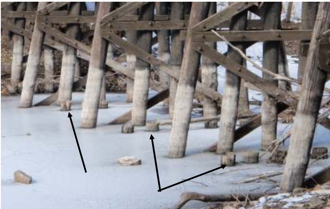
Photograph of the base of the wooden trestle bridge west of the McFarlane Bridge at low water showing the rows of original post bases just visible above the water and in rows alongside the replacement posts.
