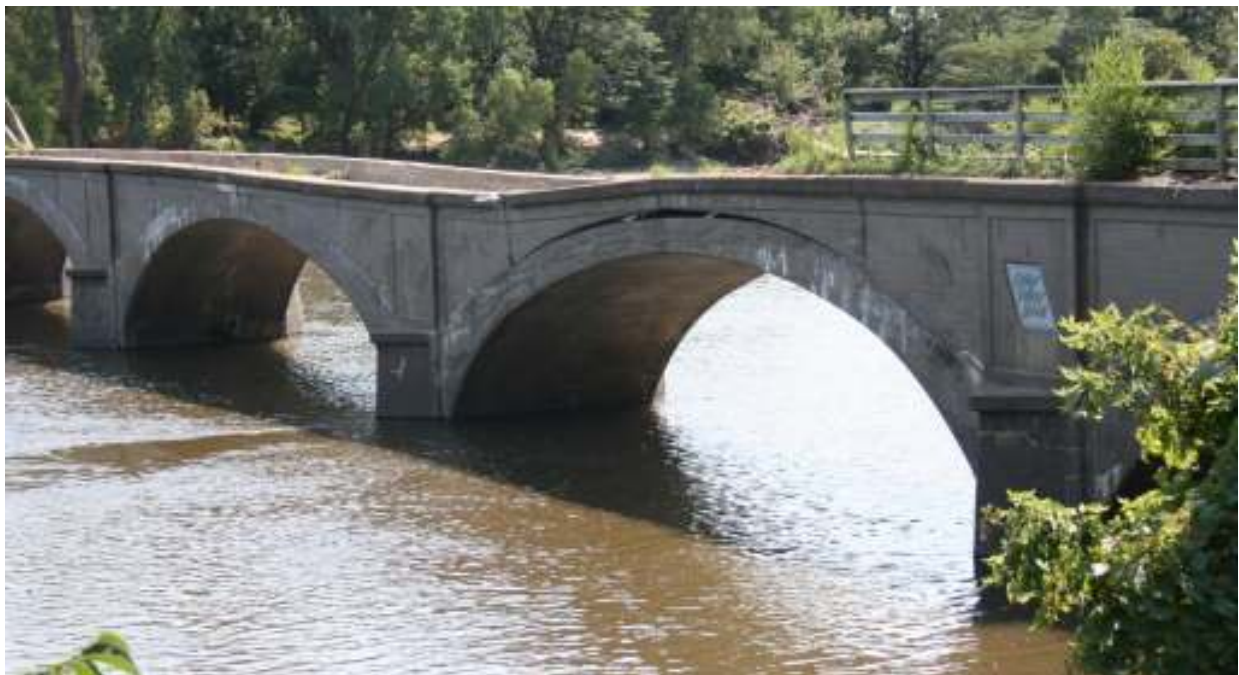
Damage to Evansdale Bridge following 2008 flooding. Photograph taken by FEMA/DHS.
