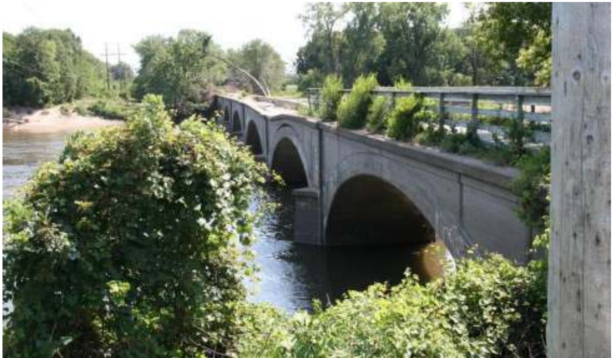
View of Evansdale Bridge following 2008 flooding. Photograph taken by FEMA/DHS.
