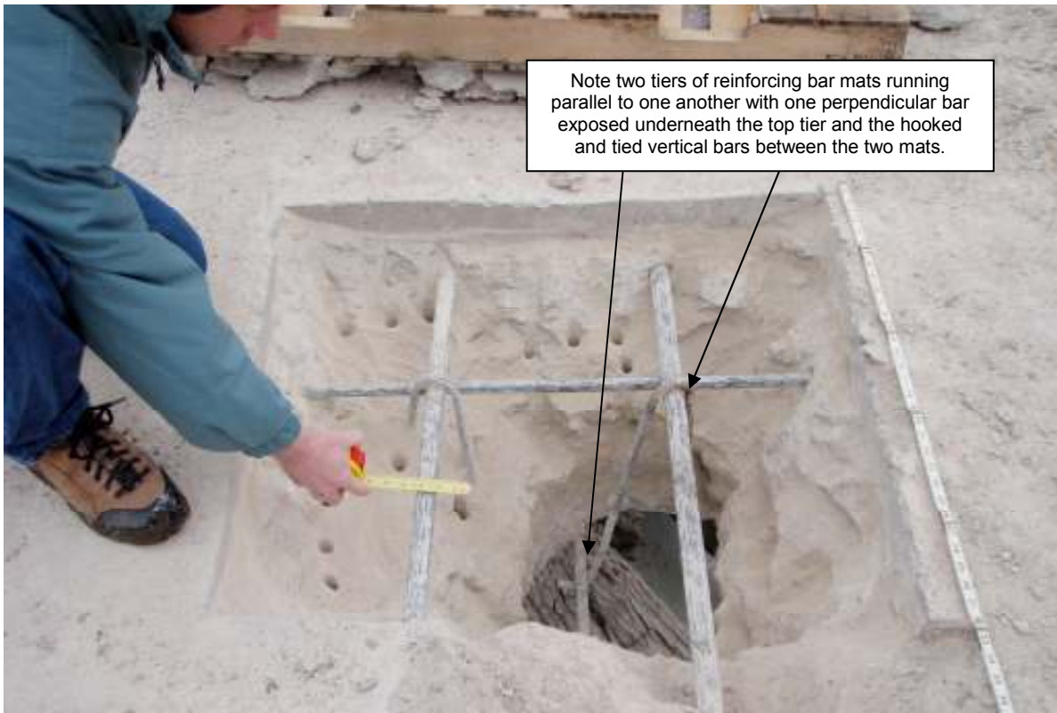
Test pit excavation in top of arch on McFarlane Bridge. Date of photograph: 9 February 2012
