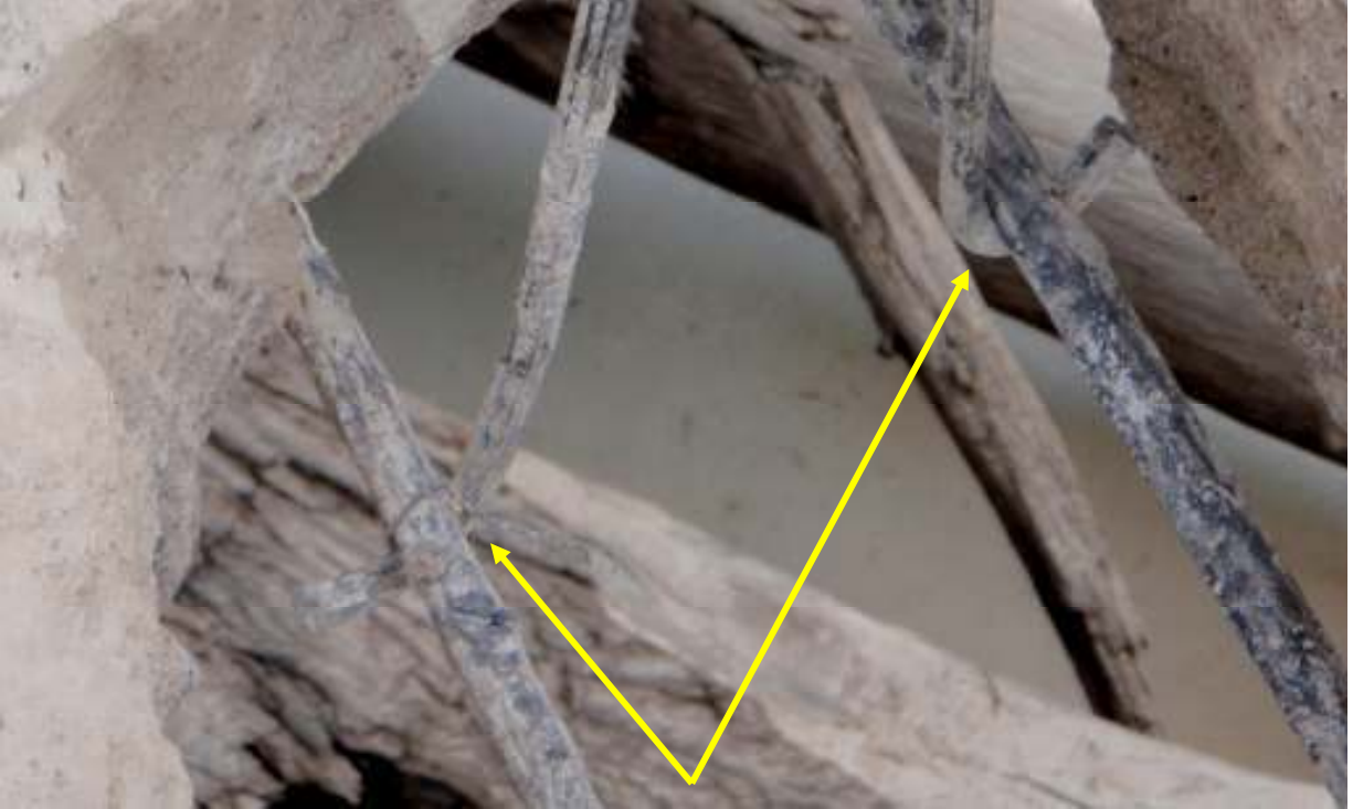
Detail of vertical bars where hooked and tied into the bottom mat of horizontal bars with wire twists.
